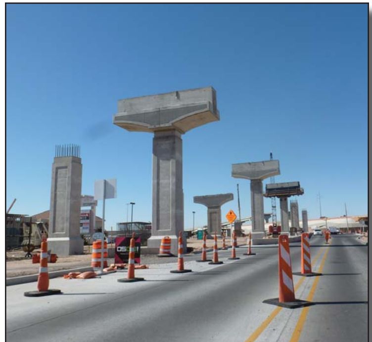
Above: Formwork for the columns of both north and southbound direct connectors.
