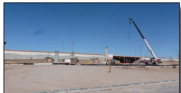
Below: During the middle of March crews were just beginning to form bents at the crossing of LP 375. Looking west at the intersection of Zaragoza and LP375.
