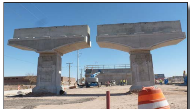
Above: Abutment construction in background, with both SB & NB Bent 2 in foreground, looking east.
