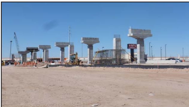
Below: Zaragoza area construction as seen from the future north bound frontage road, looking west. Bent rebar cage in foreground.
